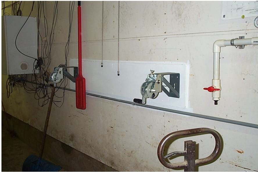
Figure 2. Pit plug pulling winch system in alleyway. There are two winches operating two separate systems in two different rooms.
